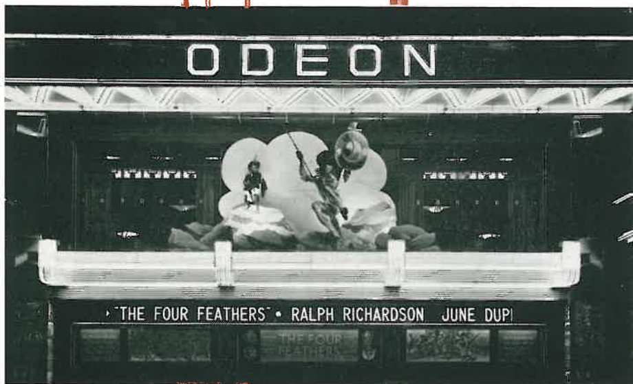
Above: The first 'all-white' high voltage fluorescent installation of cold-cathode tube type at the Odeon cinema, Leicester Square, London, 1939. Background: A Mole Richardson studio spotlight using high-brightness mercury vapour lamps. This type of unit was one of the earliest to be employed in conjunction with mercury lamps for filming.
